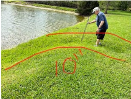
West side of lower N/S arm of Pond #3 at 8013 Stirling Falls. 10" deep and wide gully.
