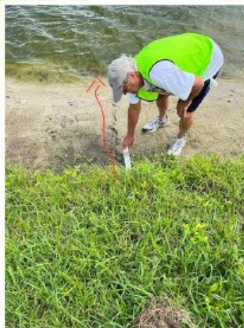
West side of lower N/S arm of Pond #3 at 8037/8033 Stirling. 25" rivulets from bottom of bank to pond. Origin??
