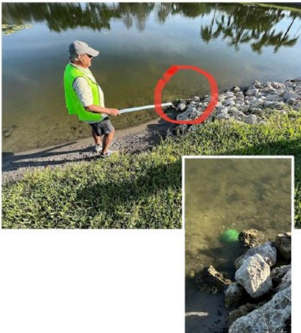
4275 Continued erosion depositing silt, partially blocking opening. Riprap slipping down slope into the pond.
