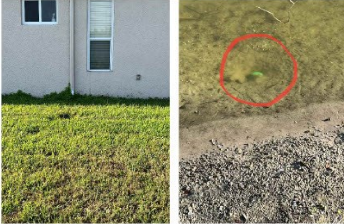
4273 buried – erosion depositing silt and partially blocking opening.
