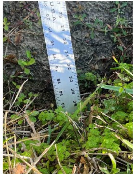
4275 12" deep cavity under bank.
